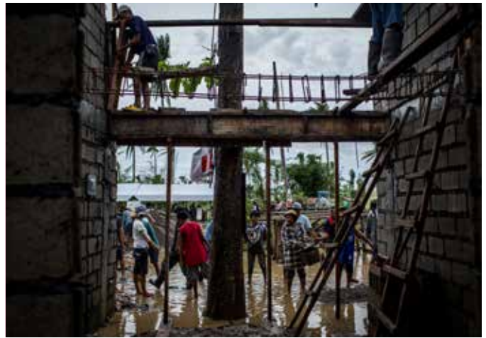
Volunteers in Tacloban working on homes for those in the “no build zone” five months after Typhoon Haiyan
