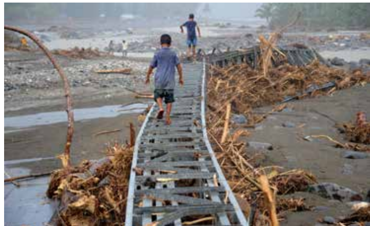
Boys play on a destroyed bridge in southern Mindanao after Typhoon Washi in December 2011
