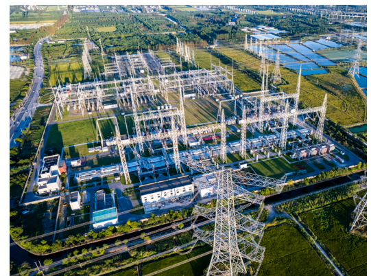
Aerial view of electricity pylons and a big electrical substation at Shanghai city, China (Getty Images)
